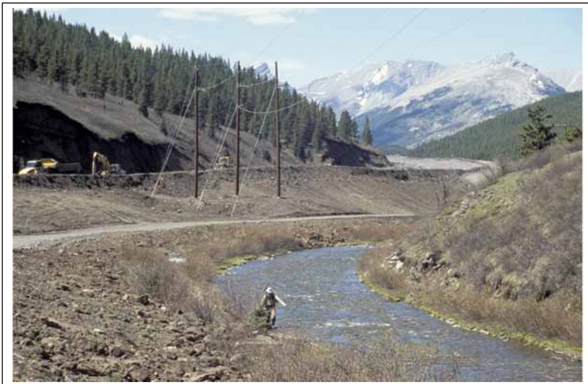
Haulroad development: clearance of riparian habitat along McLeod R., a Harlequin duck breeding stream.
