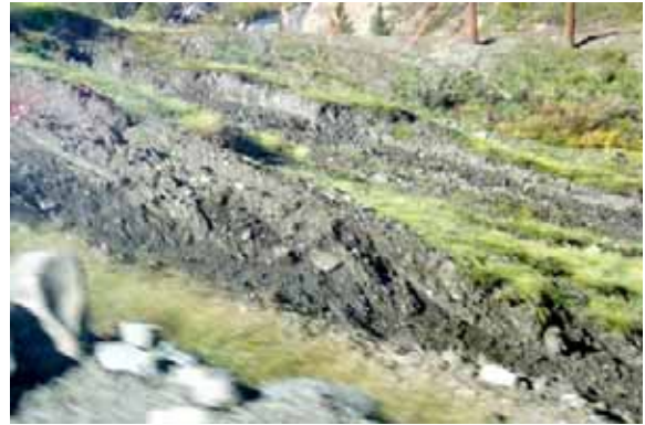
Slumping of slope below haulroad. Sept. 2005
